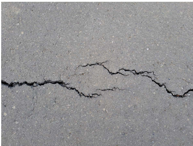
Figure 3. Two cracks circulate each other and tend to meet at right angles.
