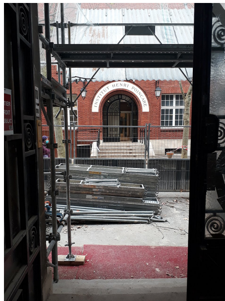
Figure 4. Entrance of Borel’s building seen from Perrin’s building door during refurbishment work, 4 March 2022.
